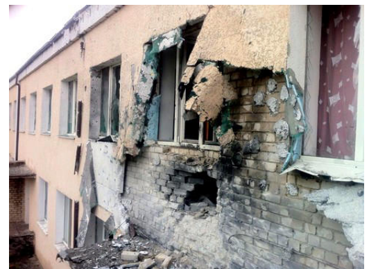
Damage at Slavyansk Children's Home
